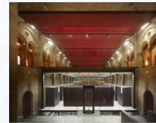
Marenostrum, Barcelona Supercomputing Centre (Barcelona)
